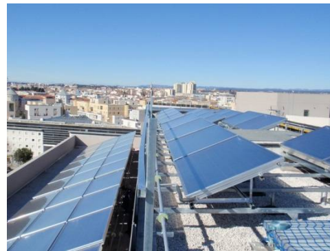
Solar collector fields in drainback mode
