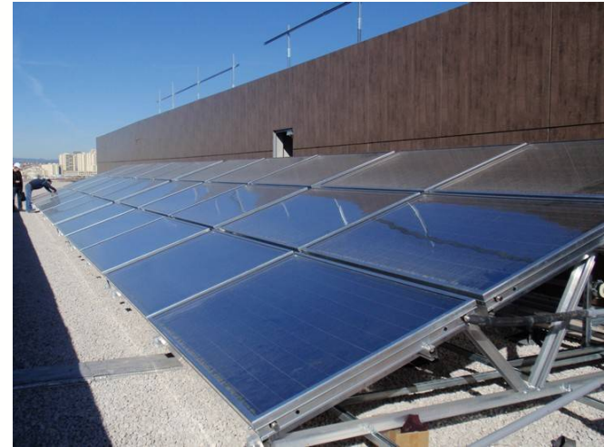
Picture of the collector field
