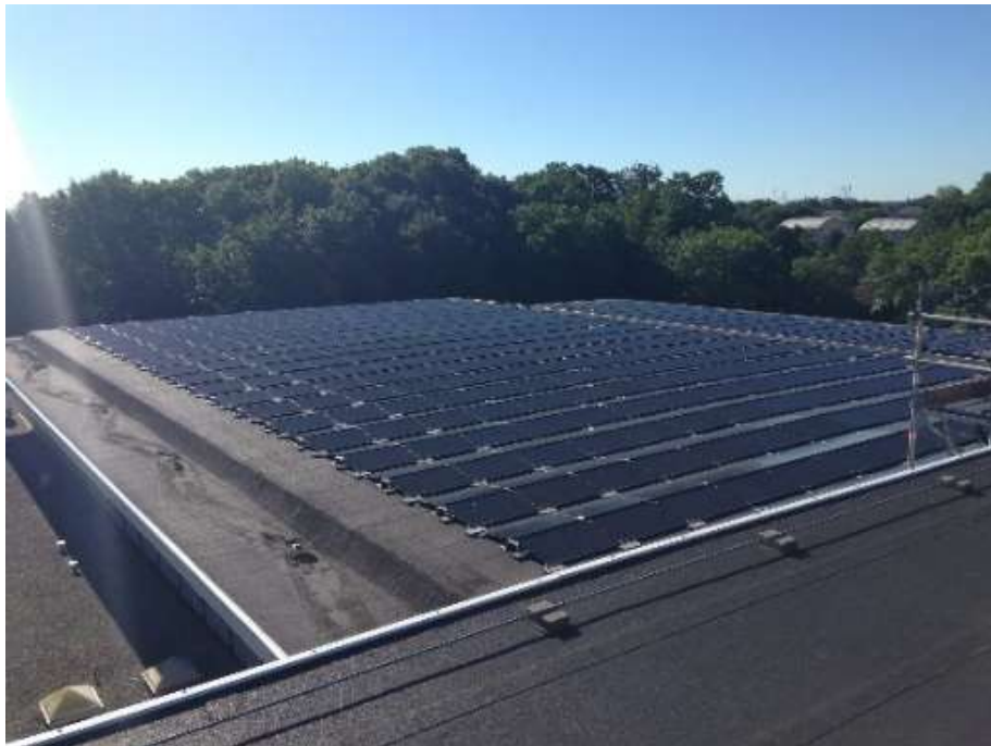
Figure 3 Photo of the PV installation on the cultural heritage site in Kildeskovshallen.
