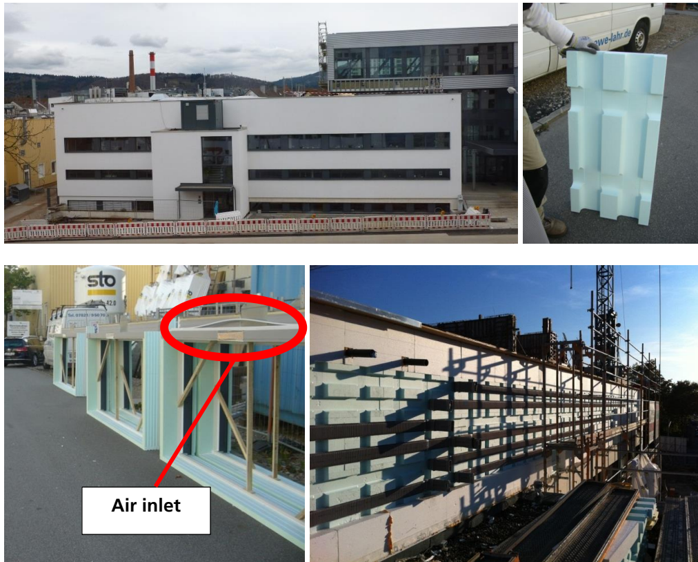
Figure 50: Retrofitted façade of the demonstration building GER04, façade and window elements for the integration of the ventilation system and building during construction [34].
