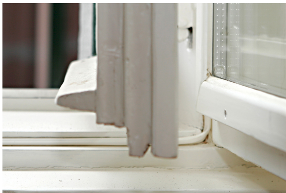
Fig. 5.2: Rebuilt double windows ( U_w reduced 2.7 to 1.35 W/m 2 K) in 141 Irding. (Photo: Hegedys & Ull/Hofer)
