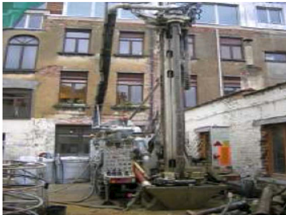
Fig. 2.11: Drilling for heat, 251 ATC Brussels (Brochure: J. Desmedt, J. Cre, W. Hilderson)
