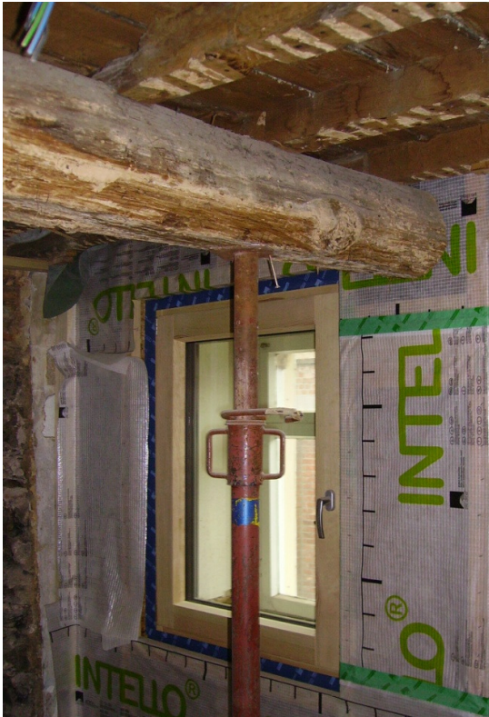
Fig. 3.1: Interior insulation of the street façade 222 ROW house in Eupen BE ( Brochure: Wouter Hilderson & Johan Cre )
