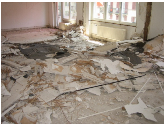
Fig 2.13: Joys of renovation, new floor plan layout. 416 APT Zürich ( Brochure: Nadja Grischott & Nadia Mastacchi )
