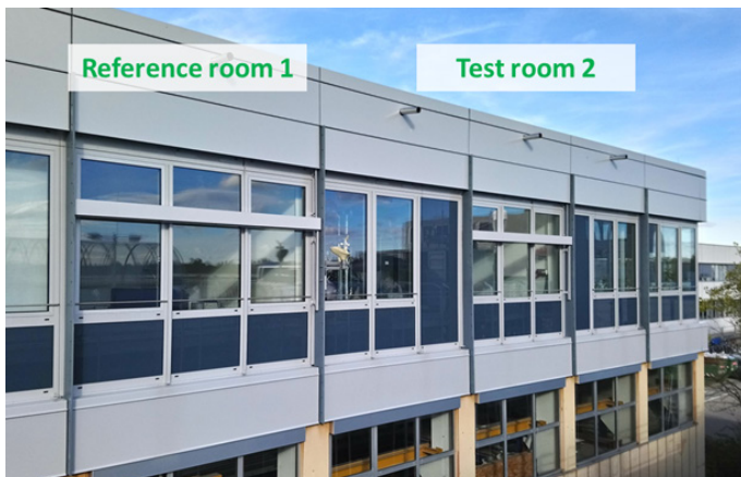
Figure 2. An exterior view of the lab. The facades of both the reference and test room can be seen in the picture.
