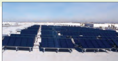
▲ Flat plate collectors used to produce solar heat for soft drink production in Arizona, USA.
