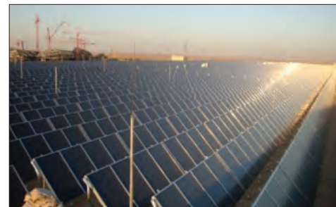
▲ Figure 1. Overview of the university's 36,305 m 2 roof mounted solar thermal collector field on a huge warehouse. (Source: Millennium Energy Industries)
