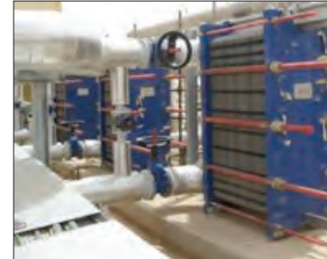
▲ Figure 4. Collector loop to the district heating network plate heat exchanger. (Source: AEE INTEC)
