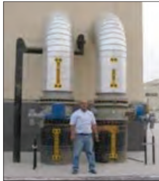
◀ Figure 5. Supply and return line of the district heating network. (Source: AEE INTEC)
