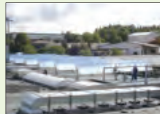
▲ P3 Pilot Plant at Alanod in Ennepetal, Germany
