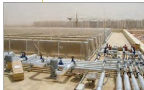
▲ Figure 2. Sectional view of the roof mounted solar thermal collector field showing the solar thermal collectors including the steel support construction and the piping for the solar primary loop. In the background is the skyline of the university campus. (Source: AEE INTEC)
