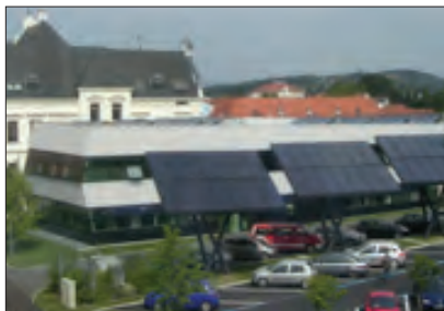
▲ Solar heating and cooling installation at the Town Hall in Gleisdorf, Austria (304 m 2 flat plate collectors connected to 35 kW Yazaki chiller WFC 10 and a desiccant evaporative cooling system).
