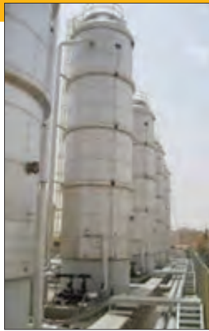
◀ Figure 3. Six storage tanks of 150 m 3 for load compensation purposes are attached to the solar supported district heating network. (Source: AEE INTEC)
